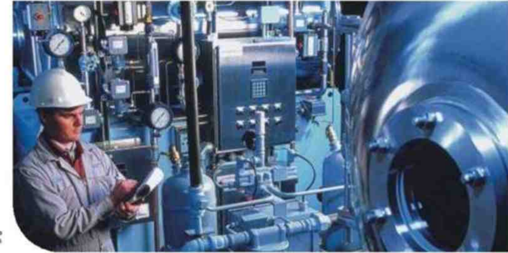
Typical application for type LTP conduit and fittings as used on machines.
